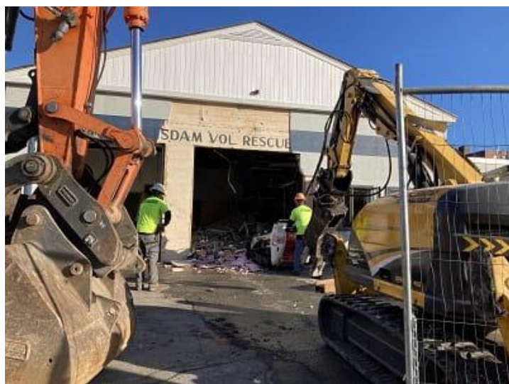
Signage from years past is uncovered during demolition of the Materials Management office.
