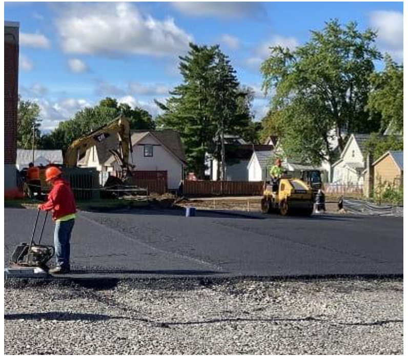
Paving is underway in the CPH parking lot expansion off Grove Street. (9-1-22)
