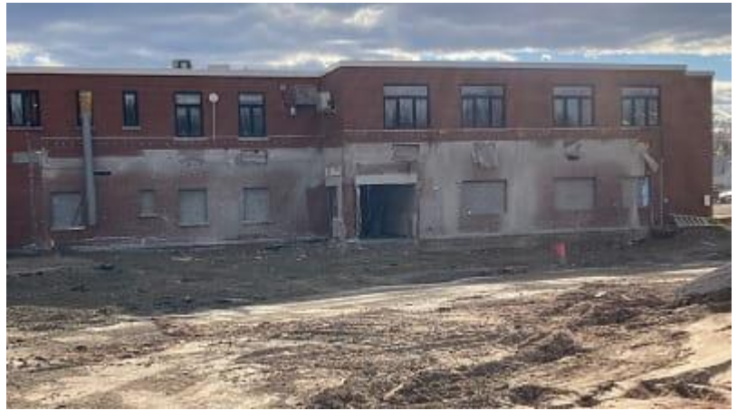
All that remains of the former main entrance. (11-7-22)
