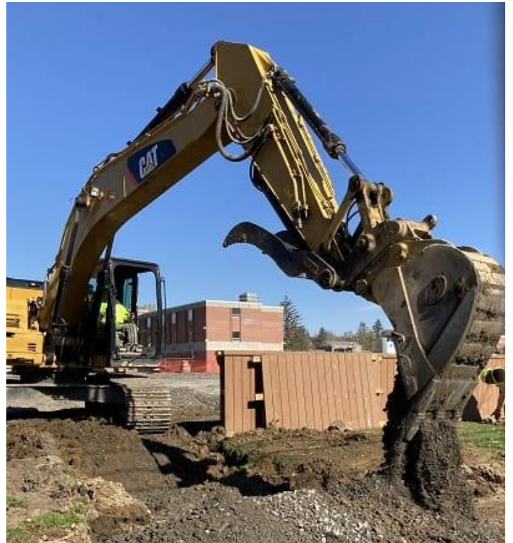
Backhoe work off Cottage Street at the former back lot near the ER. (10-21-22)
