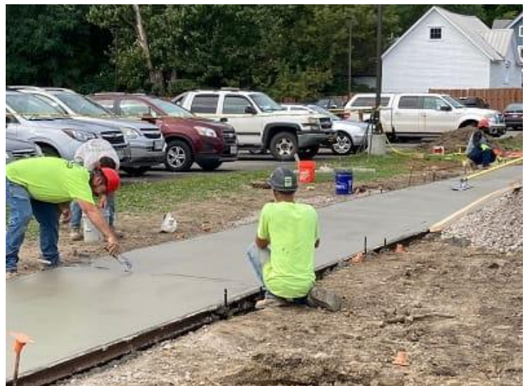
A new sidewalk is poured and prepped on the south side of Cottage Street. (9-7-22)
