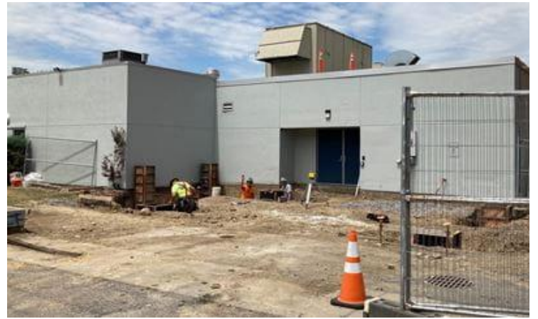
Work is underway on the temporary entrance on the Cottage Street side of the Hospital. (7/11/22)
