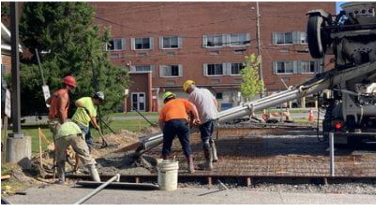
Cement is being poured for the new compactor pad at 25 Cottage Street. (7/26/22)
